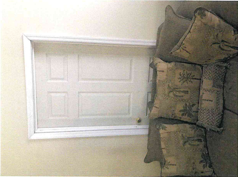
16 N Cypress - duplex conversion/unpermitted
