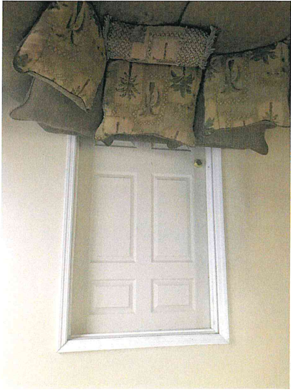
16 N Cypress – duplex conversion/unpermitted
