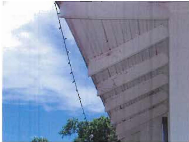
9: South Facade Roof Overhang - Note Rafter End Repairs
