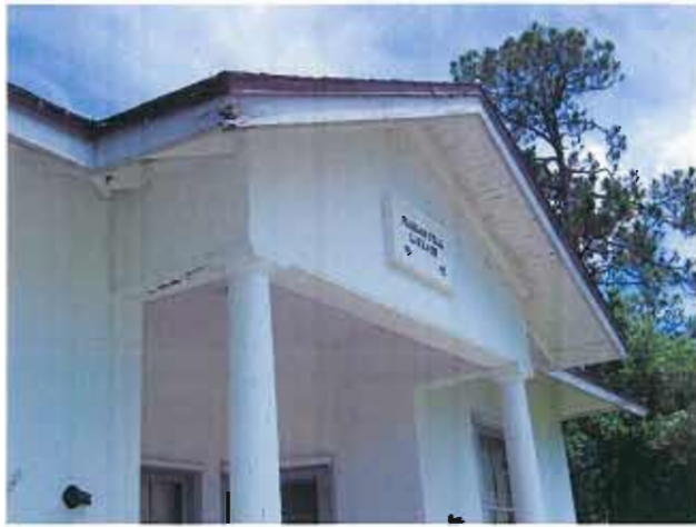
7: Principal Facade Fascia - Note Deterioration
