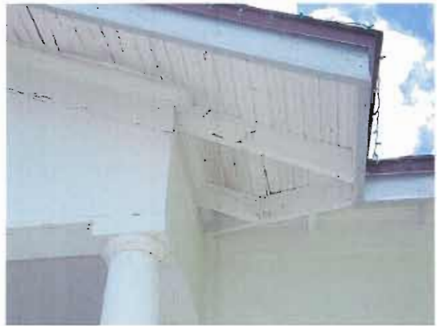
8: Principal Facade Fascia - Note Rafter End Repairs
